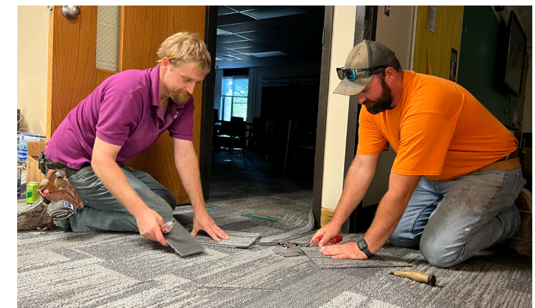
Brothers Sawyer Long, 2011 Sherrard graduate and Mason Long, 2005 grad work on carpet installation with Long's Carpet, based out of Rock Island. The company employs several Sherrard alum who have worked on the building. The brothers still live in the school district and have children that attend. Cala Smoldt
