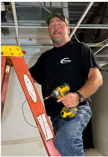
Mike Iverson (above), Crawford Company, '88 Sherrard graduate, worked in the rafters of the new science lab. Cala Smoldt
